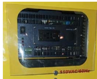
AC End (Inverter - switch is on left.)
