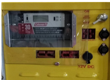
DC End (Charge Controller on left.)
